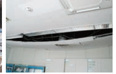
A collapsed ceiling at the Shirakawa Plant
