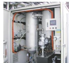
Waste Liquid Treatment Equipment
