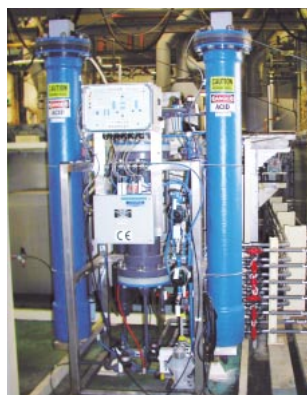
Acid Recovery Equipment
